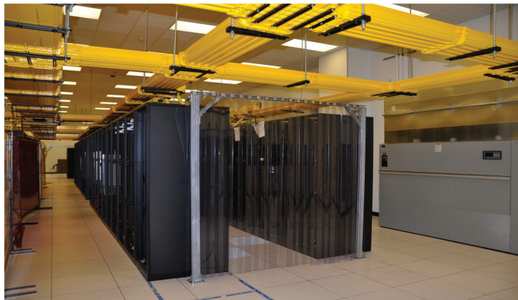
Cold aisle refrigerator curtains
