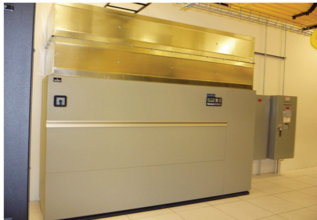
CRAC with an air return extension
